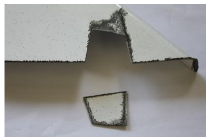
Fig. 6 Sample with blisters defect
