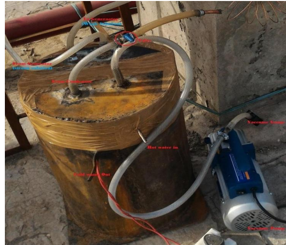
Fig.4 Evaporator and Absorber Tank
