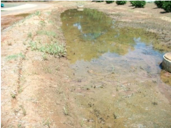
Fig. 5. Ponded water on the biofilter surface observed after rainfall (the vegetation cover is very poor indicating likely serious compaction).
