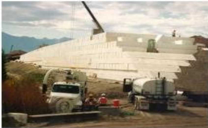
Fig2. Typical geofoam embankment construction on the I-1 reconstruction project in Salt Lake City
