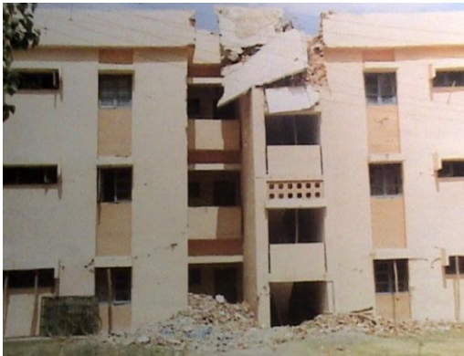
Fig.7. Damaged building at Agriculture University
