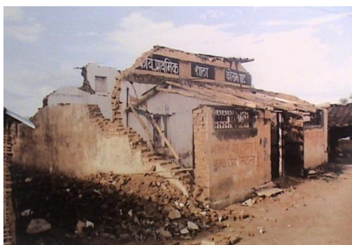
Fig 10. Damaged school building at Kosamghat (Centre of 1997 EQ)
