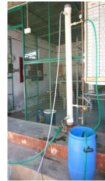
Fig.1 Photo of Water Scrubber
